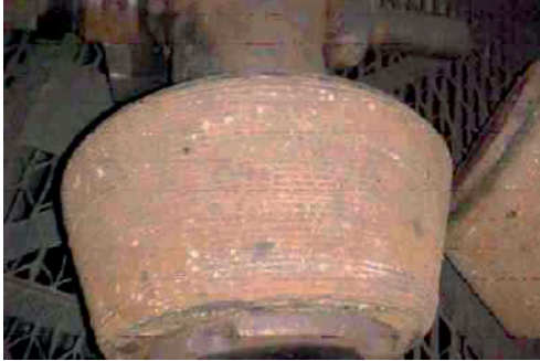
Coal Mill Grinding Roll
