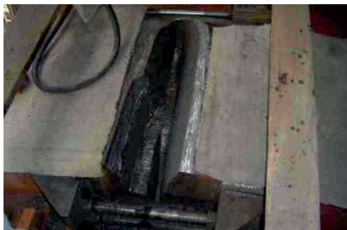
Gouging Kiln Girth Gear
