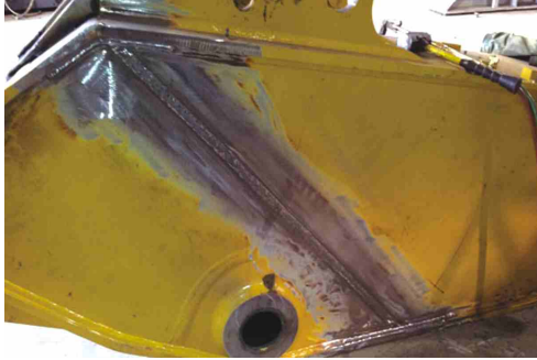
Excavator Boom Crack
